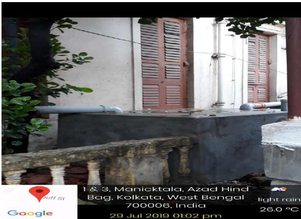
Fig E:Reservoir of roof water harvesting
