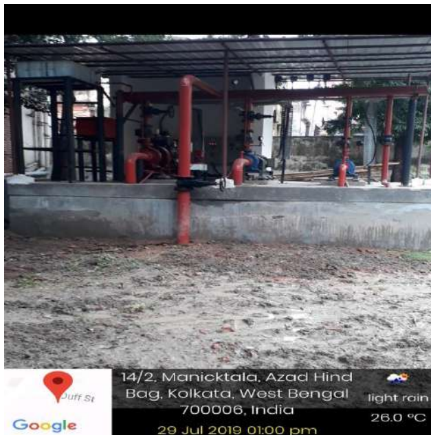
Fig F: Fire fighting system in main campus
