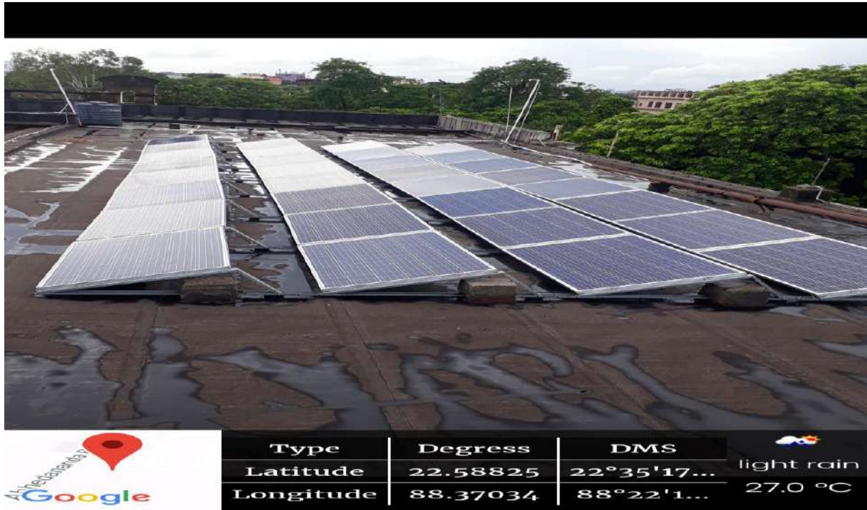
Fig B: Solar panels on roof top
